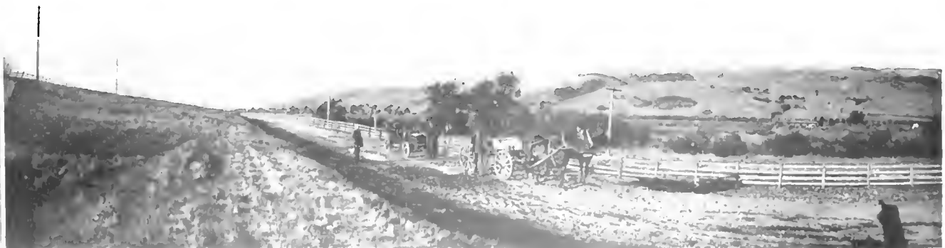
IMPROVING A ROAD IN SANTA CLARA COUNTY, CALIFORNIA, WHERE GRAVEL BEDS PREDOMINATE.
